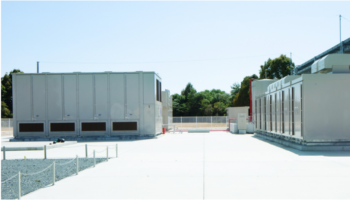
Large-capacity power storage system (Yamaguchi Plant)
