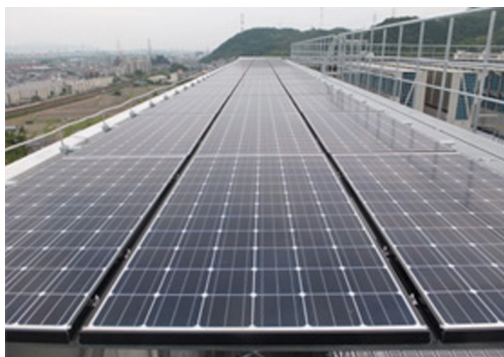
Solar panels at the Minase Research Institute
