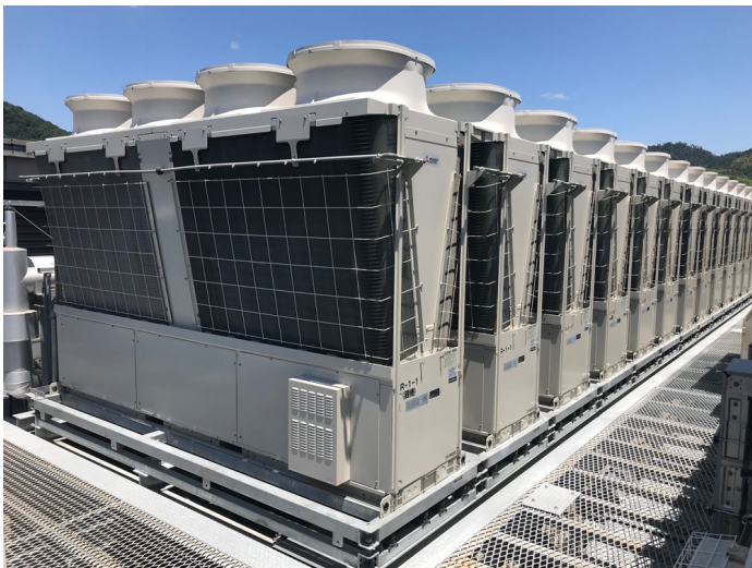
Module-type heat pump chiller (Minase Research Institute)
